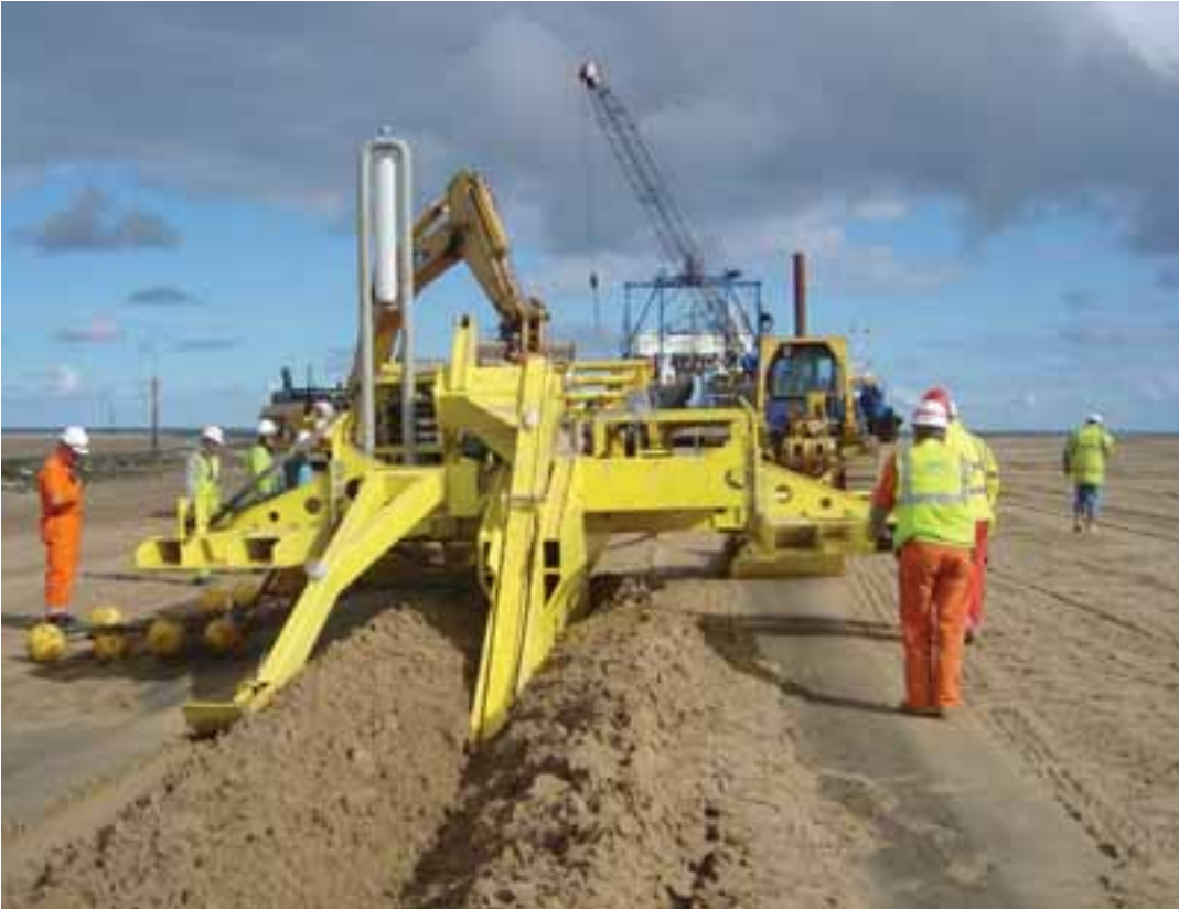
Figure 3.13: Conventional Narrow Share Cable Plough Burying a North Hoyle Offshore Wind Farm Export Cable
